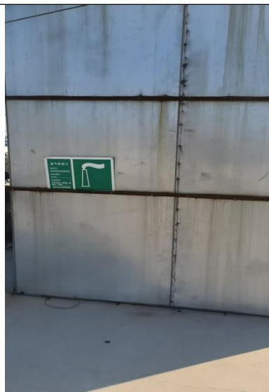
FQ-01 排气筒及环保标牌
