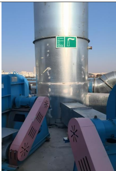
FQ-02 排气筒及环保标牌
